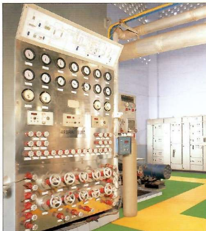
300 cu.m/hr Oxygen Plant area
