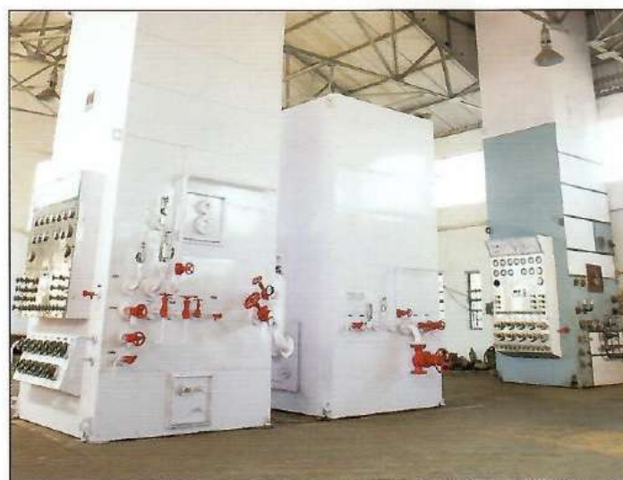
1000 Cu.m/hr Oxygen Column
