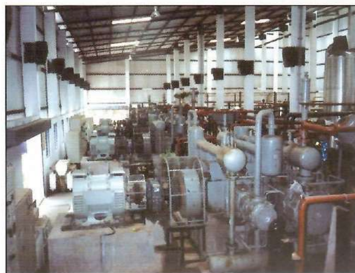
Air Compressors - 60 tpd Plant
